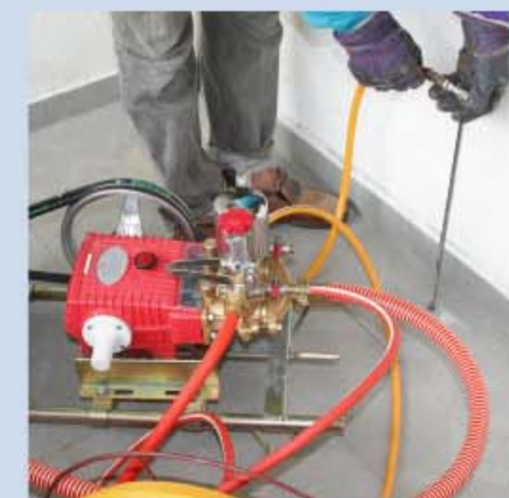
Premise 200 SC injected through slab. Each hole is filled with 5 liters solution.
